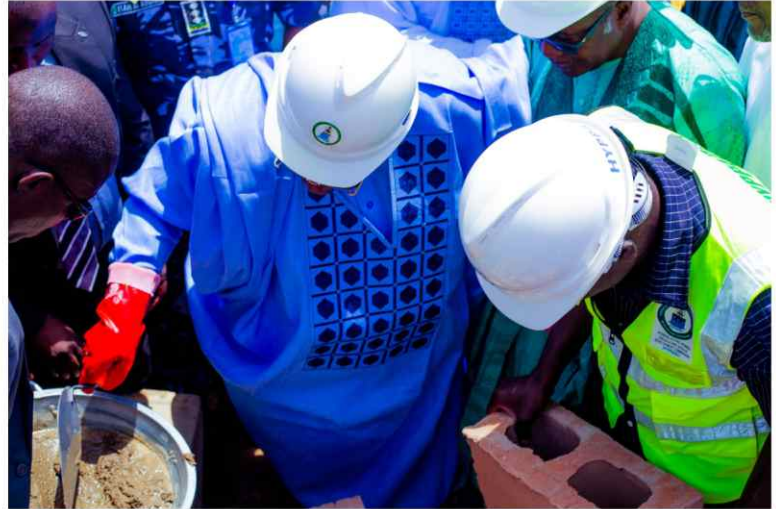
Dr. Nasir Idris performing the ceremonial foundation laying for the 30-unit resettlement housing scheme
