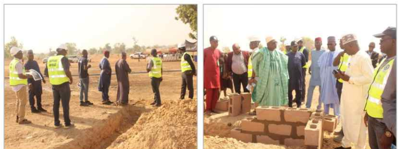
Alh. Abubakar Sadiq Yelwa supervising the on-going work of the construction of the 30 Unit resettlement scheme
