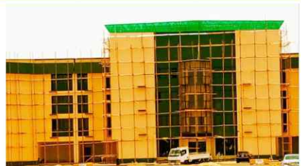
Front entrance of the ongoing construction of the Ultra modern State Secretariat complex in Birnin Kebbi
